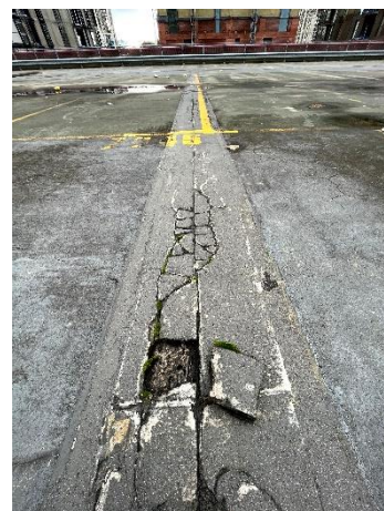
Fig. 14 – Damaged seal over joint
